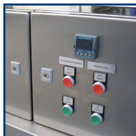
Process water temperature control via individual controller
